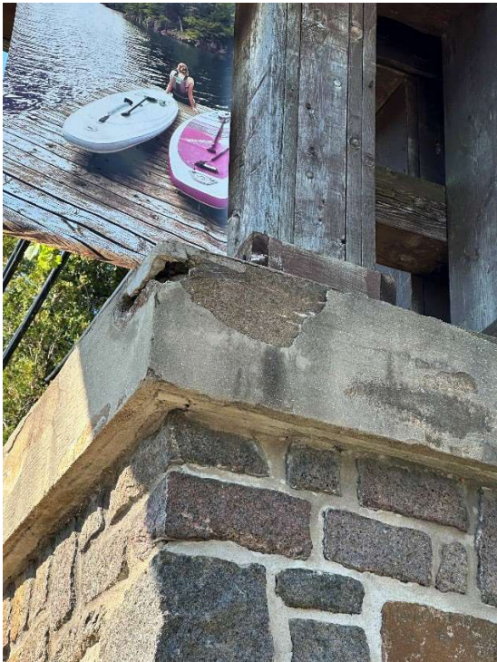
Figure 8: Delamination of concrete cap - West side, North Gate
