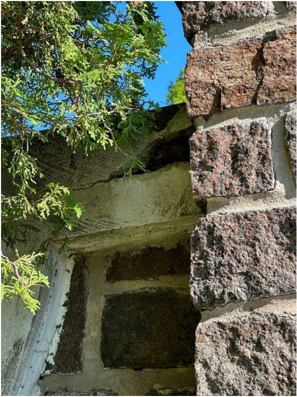
Figure 10: Hole in West concrete cap - South face - North Gate
