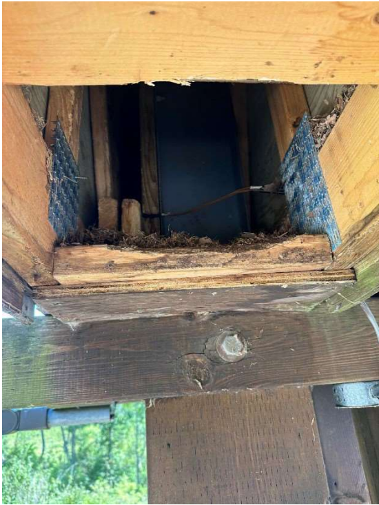
Figure 28: Debris and minor water staining inside arch - West Gate South Side
