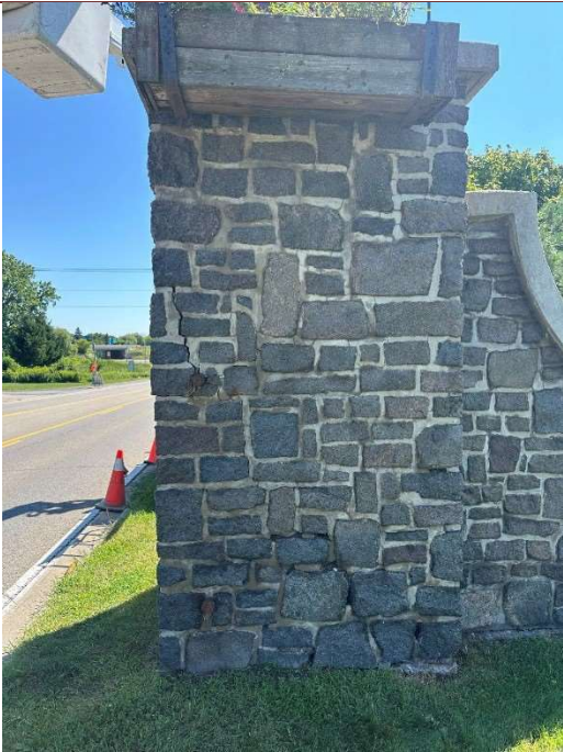
Figure 17: Step Cracking in South Support at East Gate
