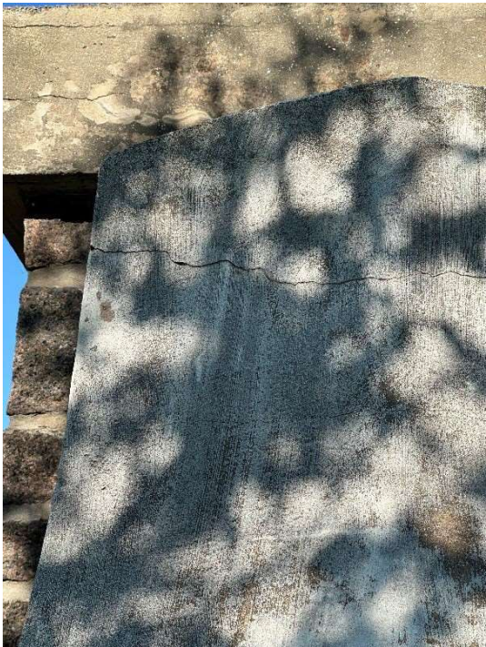
Figure 6: Minor Cracking in Wing Wall Cap
