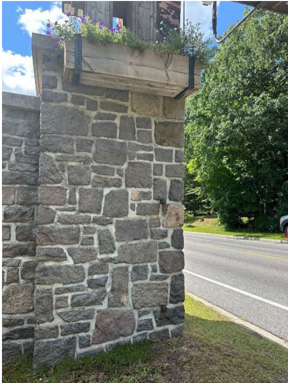
Figure 24:Old Bolts in South Support - West Gate
