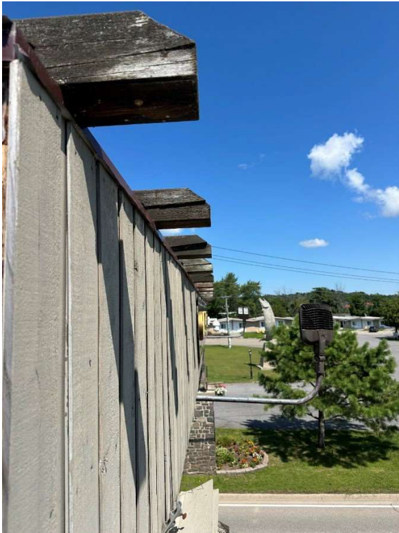
Figure 20: Sun damaged cladding and outriggers - East Gate
