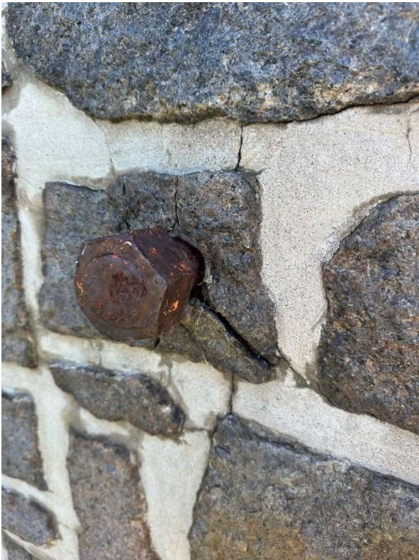
Figure 16: Broken block at old bolt location - East Gate Support
