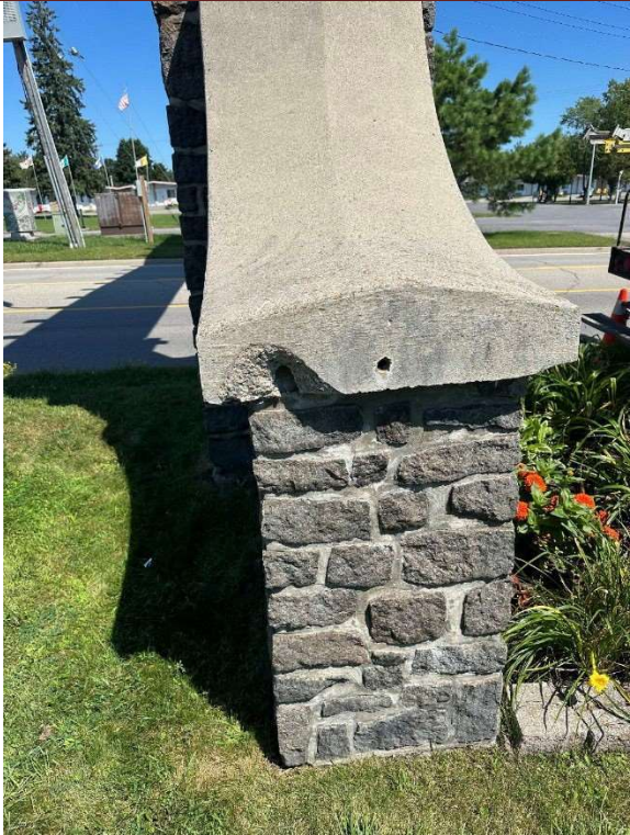
Figure 19: Damaged concrete cap at South Wing Wall - East Gate
